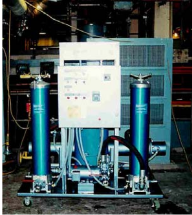
Coalescer in use at Power Plant on Steam Turbine Lube Oil System
